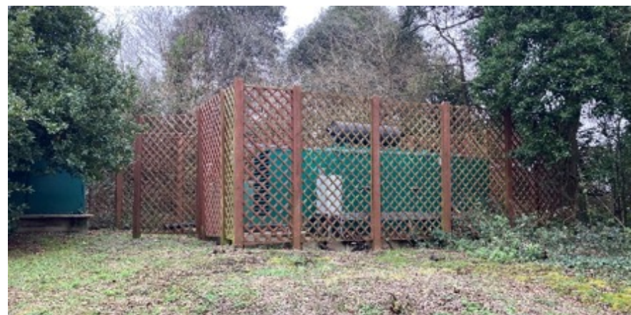
Figure 28: Plant within the grounds of Goring Hall
